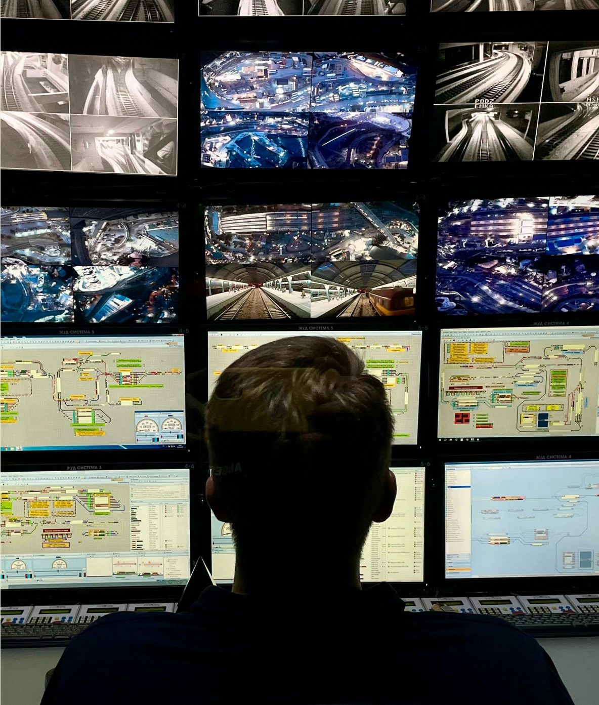
Centrally integrated 7/24 security with CCTV monitoring
